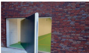
External Steel Pivot Doors as Entrance Doors
